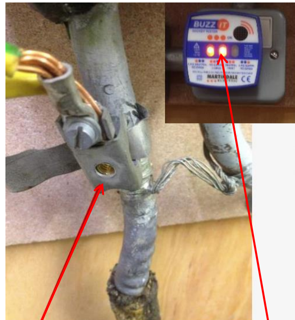
Screw missing from the earth clamp.
