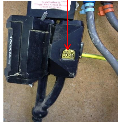
Knock out missing and the neutral-earth is exposed – do not report
