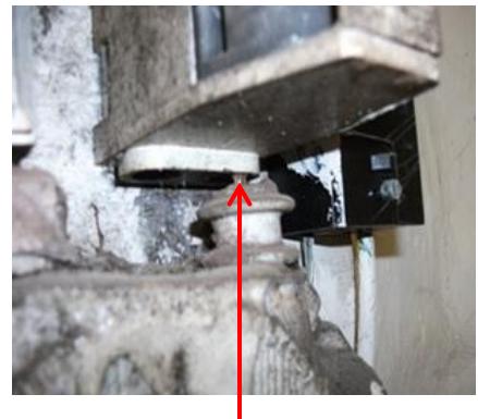
Visible bare conductors
