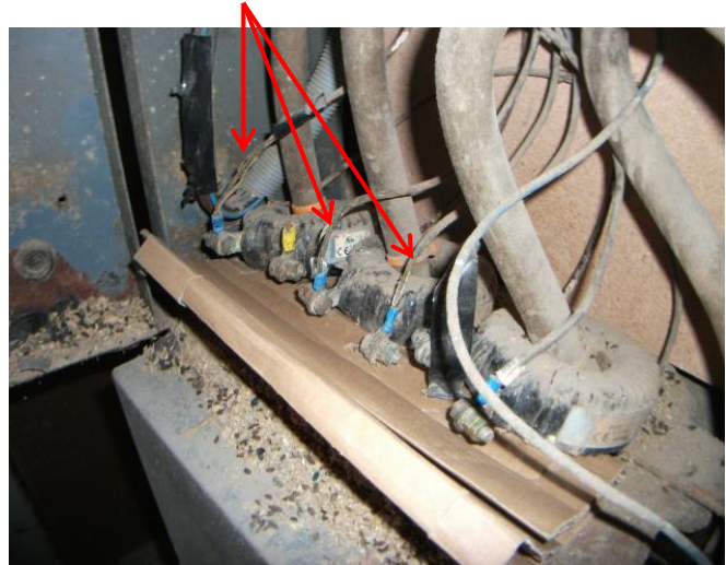
CT wiring insulation damaged by rodent infestation exposing inner conductor
