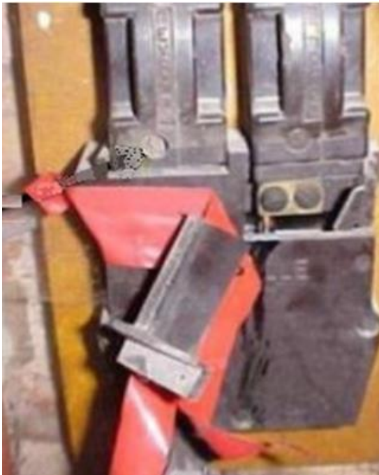
Severely damaged cut-out casing
